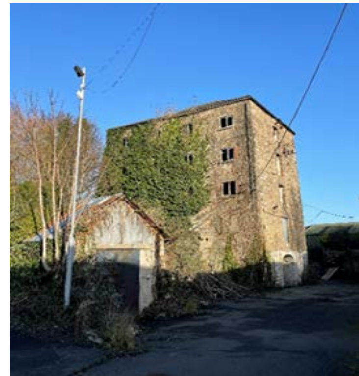
Figure 32: Current unmaintained condition
