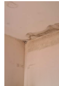
Mould in Bedroom Wall to Ceiling Junction
