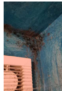
Mould in Toilet Wall to Ceiling Junction
