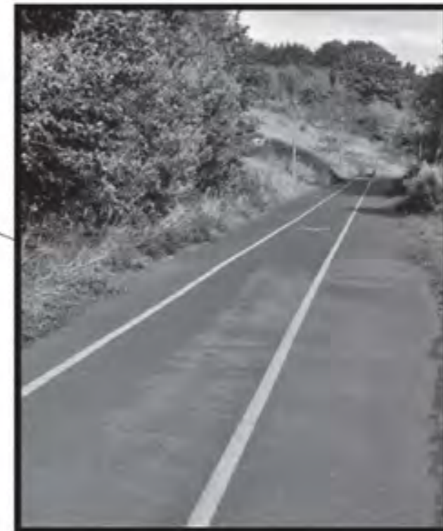
Fig 2; Leachate seeping up through the paths within the Tolka Valley Park
