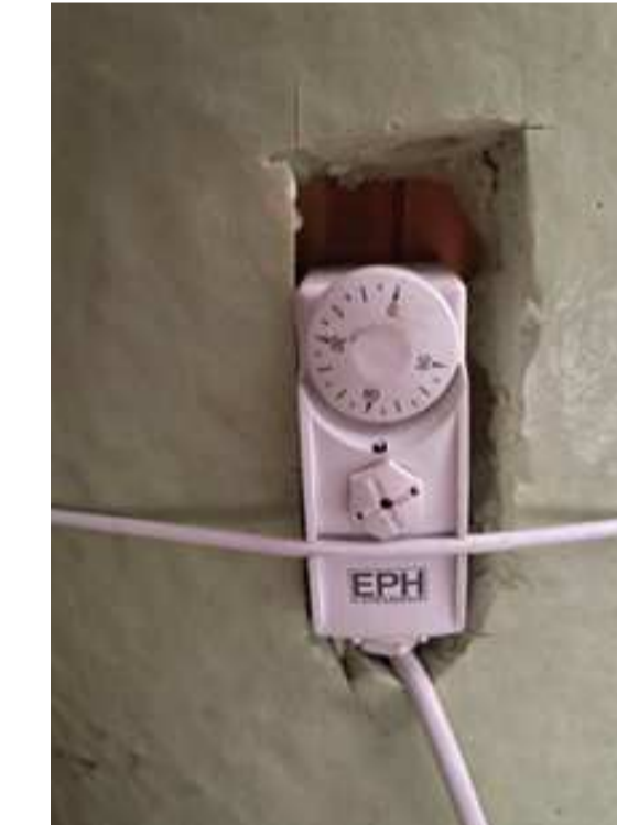
Domestic hot water thermostat controlling supply temperature @ 65°C
