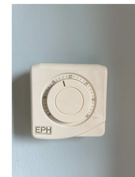
1. Thermometer in hallway to control heating, set to 18°C
