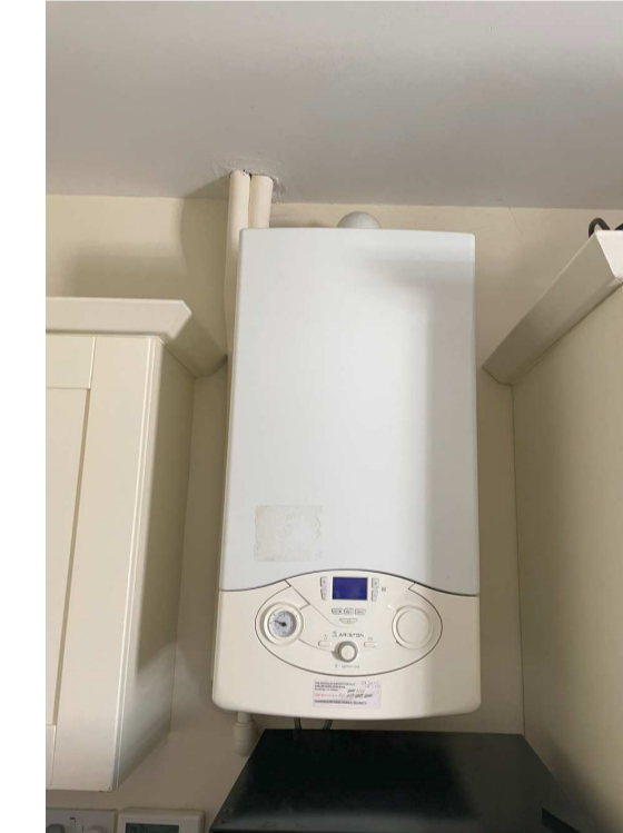
30kW Ariston Gas boiler 97.8% Efficiency Heats radiators & DHW
