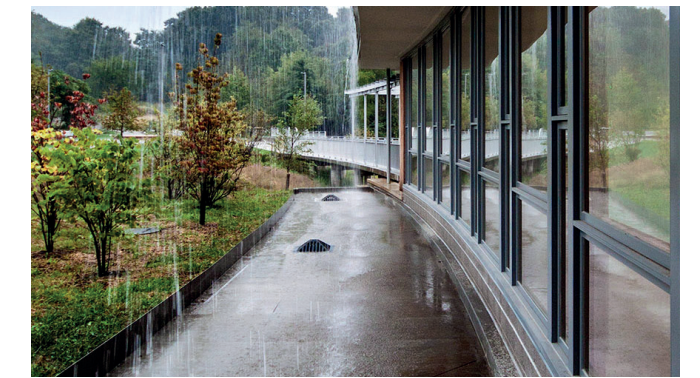
[fig 42] Roof water veil
