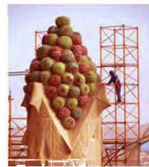
Fig.2.2.2 La Sagrada Familia - They also used original materials, such as clay tiles, to repair the roof, and they carefully documented their work so that it could be undone if necessary.
